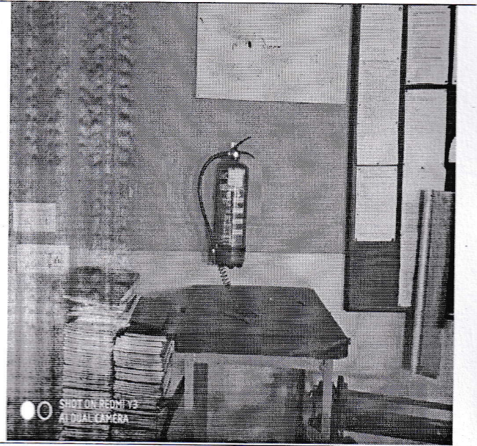
Fire Extinguisher in D-Block
