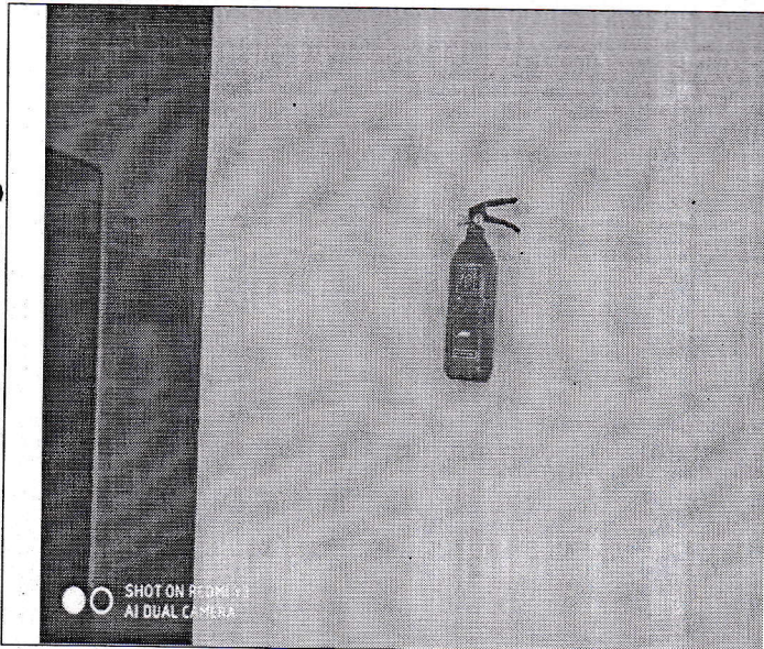
Fire Extinguisher in B-Block
