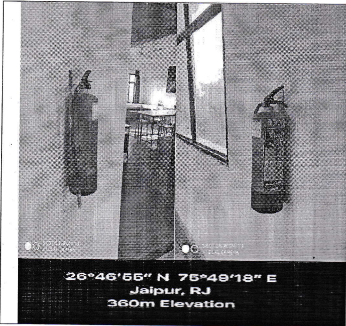
Fire Extinguisher in C-Block
